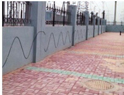
Embedded on the wall
